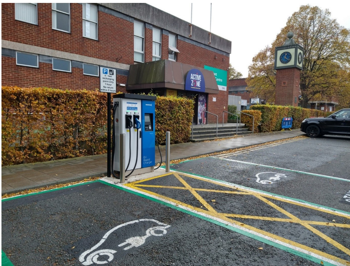
Electric vehicle charging point for taxis in Central Avenue
